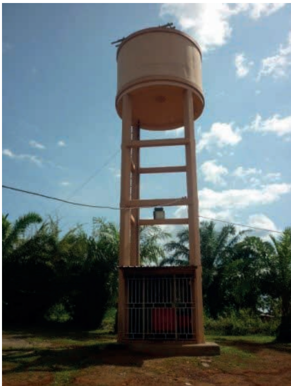
Monavebe's water tank, guaranteeing a potable water supply.
